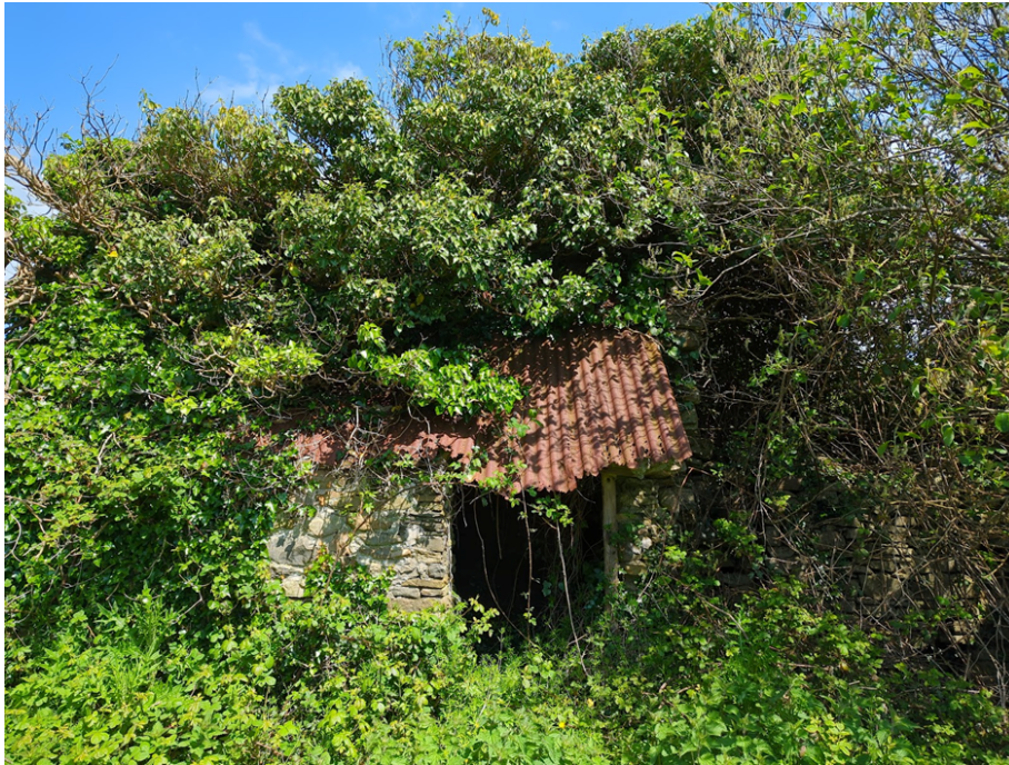
Photograph 17. Old shed in poor state of repair (Location B) within proposed development site
